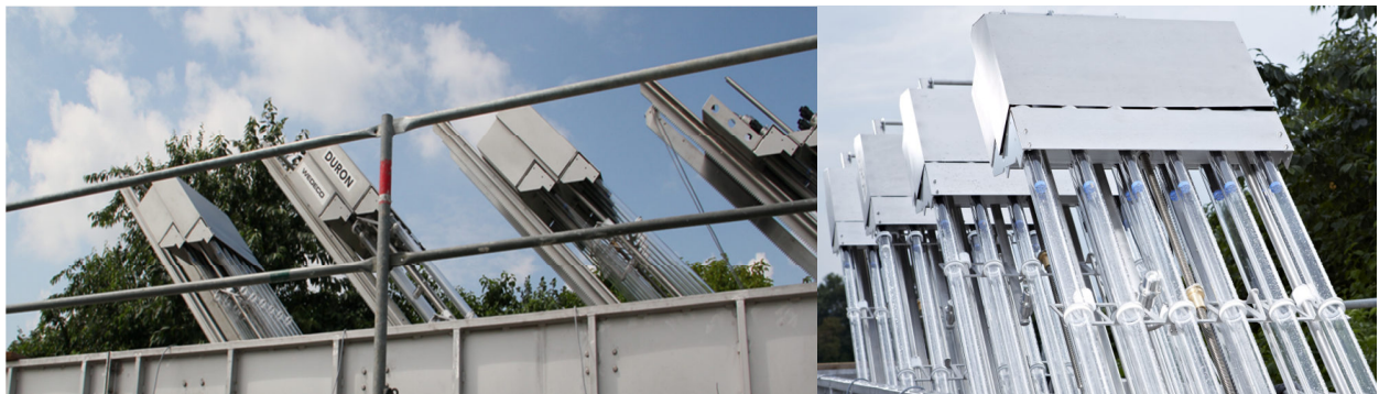
Figure 2: Wedeco Duron UV validation system
